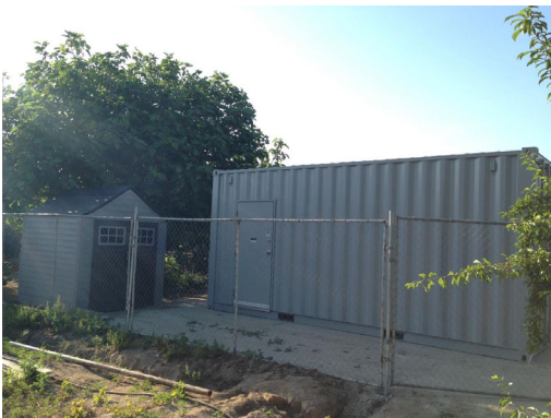
Example: Containerized Biological Treatment System
